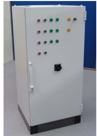
Local Control Unit
