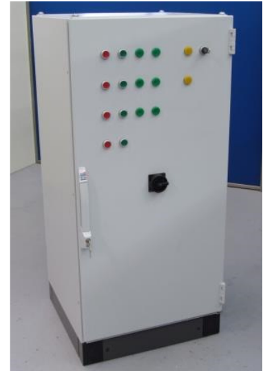
Local Control Unit
